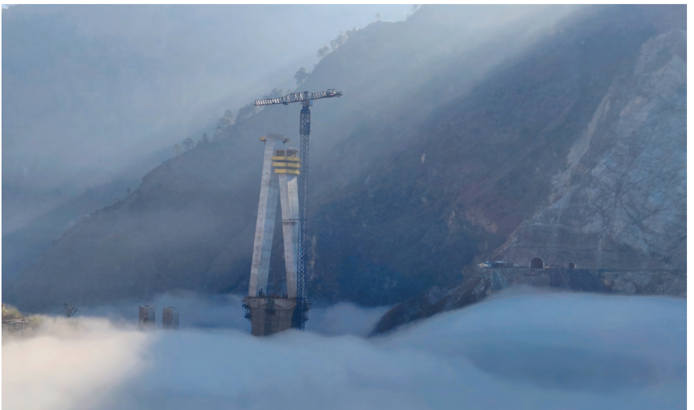
TOP AND ABOVE: To respond to the demands of the project and the challenges involved in constructing the pylon at such a remote, complex site, HCC selected a 21CM550 flat-top tower crane from Comansa. This crane model is designed to ensure optimal performance in projects where heavy loads must be moved, like those in bridge construction.
