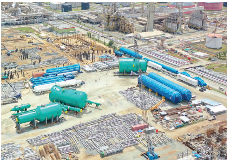
Thanks to the wide steering angle and remote control for the three self-propelled modules, the loads could be manoeuvred in the most confined spaces.
