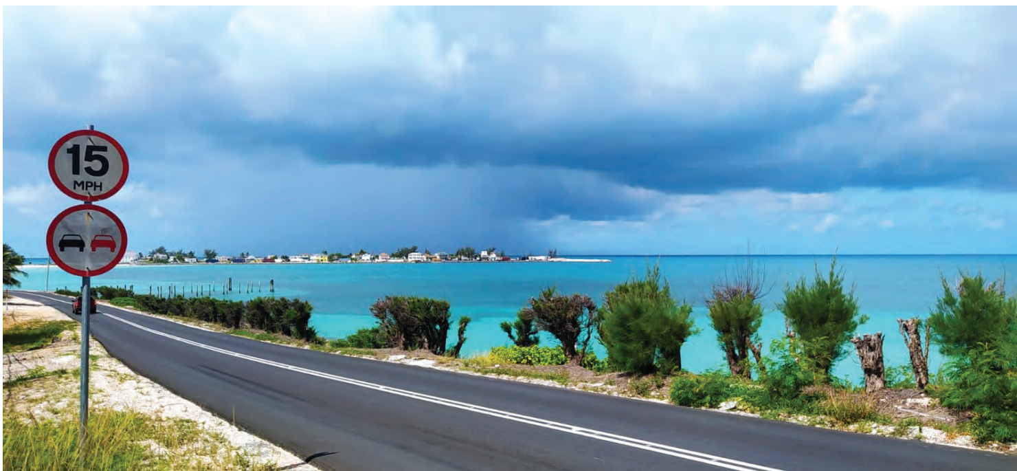
BHM Co Ltd was involved in the rebuilding of the Queen's Highway in the Bahamas. The road resurfacing and maintenance work encompassed the application of approximately 15,000 tons of asphalt mix.
